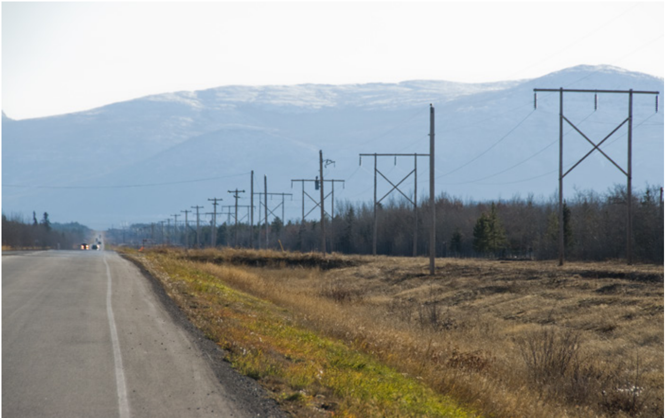
Power lines running along highway.
