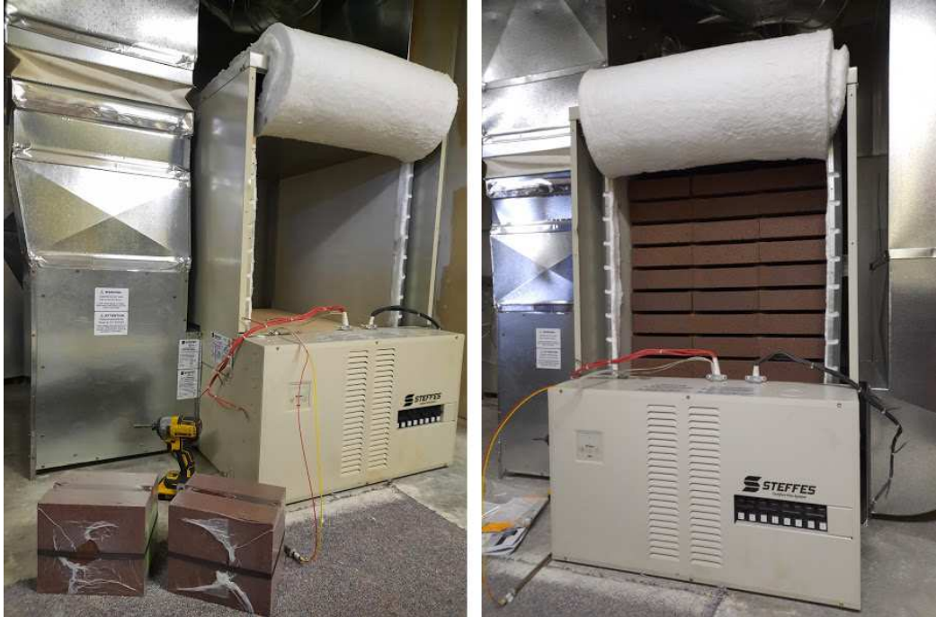
Photo: YCS's new ETS furnace being installed, before and after the unit's bricks were loaded in.
